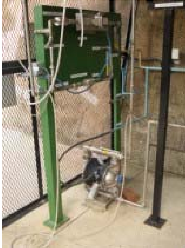
The Control Panel.
